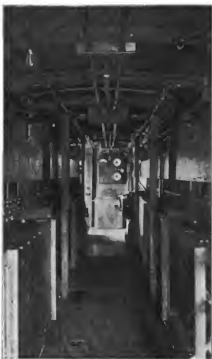
Fig. 4655. Interior View of Cab. Westinghouse A. C. Electric Locomotive.
